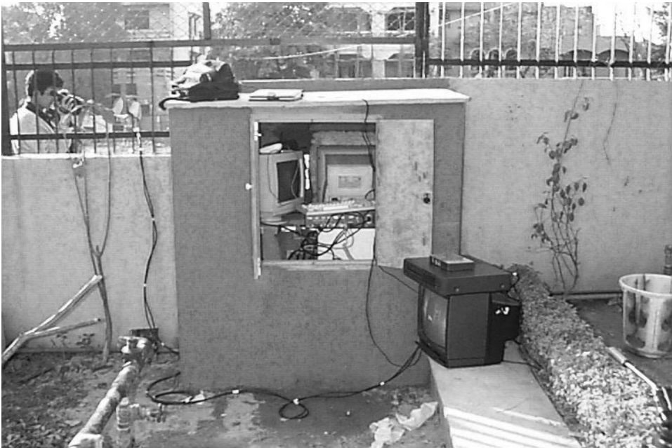
Figure 2: Construction of the kiosk housing on the office side of the wall
